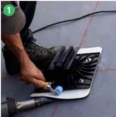
Weld one side of the base panel over a minimum width of 3 cm.
